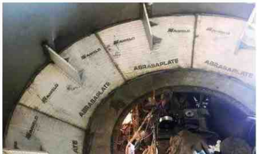
Hydropulper lined with AbrasaPlate wear plates, with AbrasaPlate-X cross hatch baffle plates
